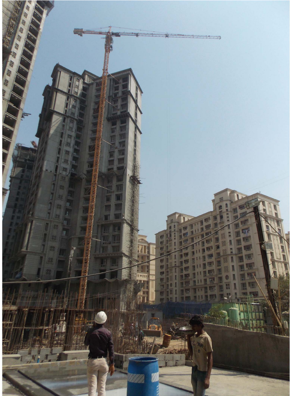
“ Clayton” (Work in progress) Rodas Enclave, Hiranandani Estate, Off. Ghodbunder Road, Thane.
